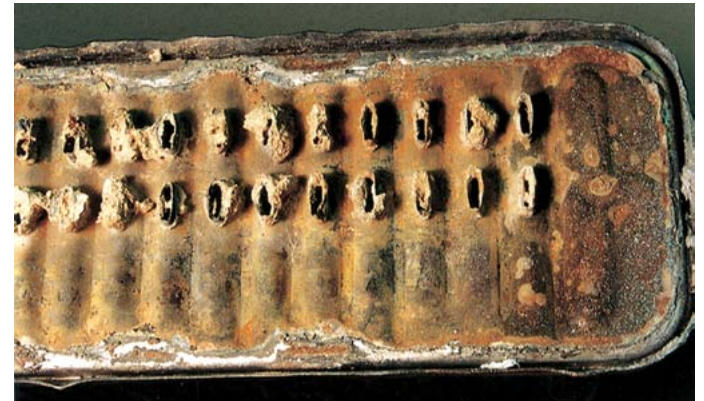
Neglected Cooling System
